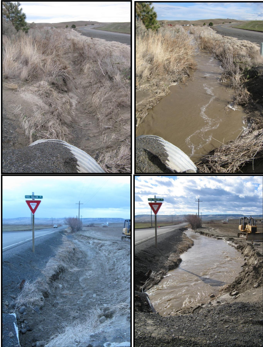
Figure C-1: Burlingame overflow ditch before and after opening. (Upper) looking upstream and (Lower) looking downstream. March 6 and 7, 2014.
